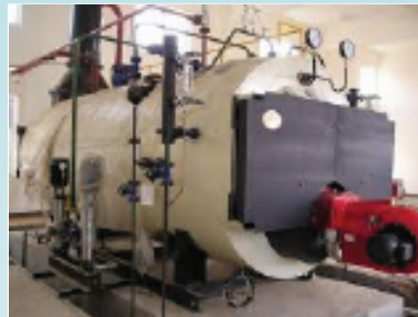
Boiler water replenishment
